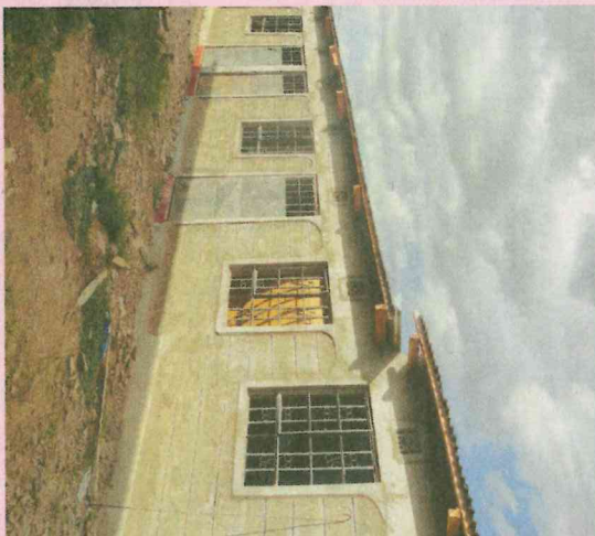
PHOTO | JOEL KAPANTE REVIA Investors are building simple houses like this one for the migrant labour force in the Mara.
